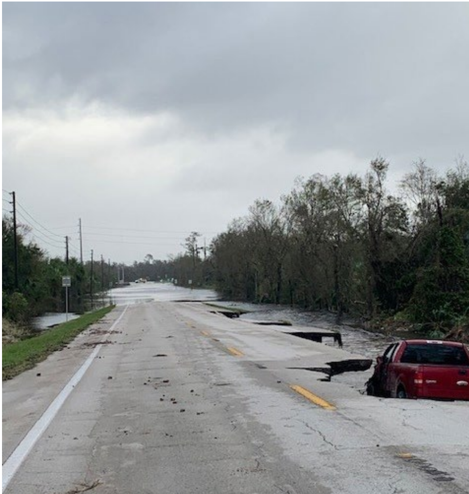
Figure 11: Severe flooding and road damage on SR 72 during Hurricane Ian
