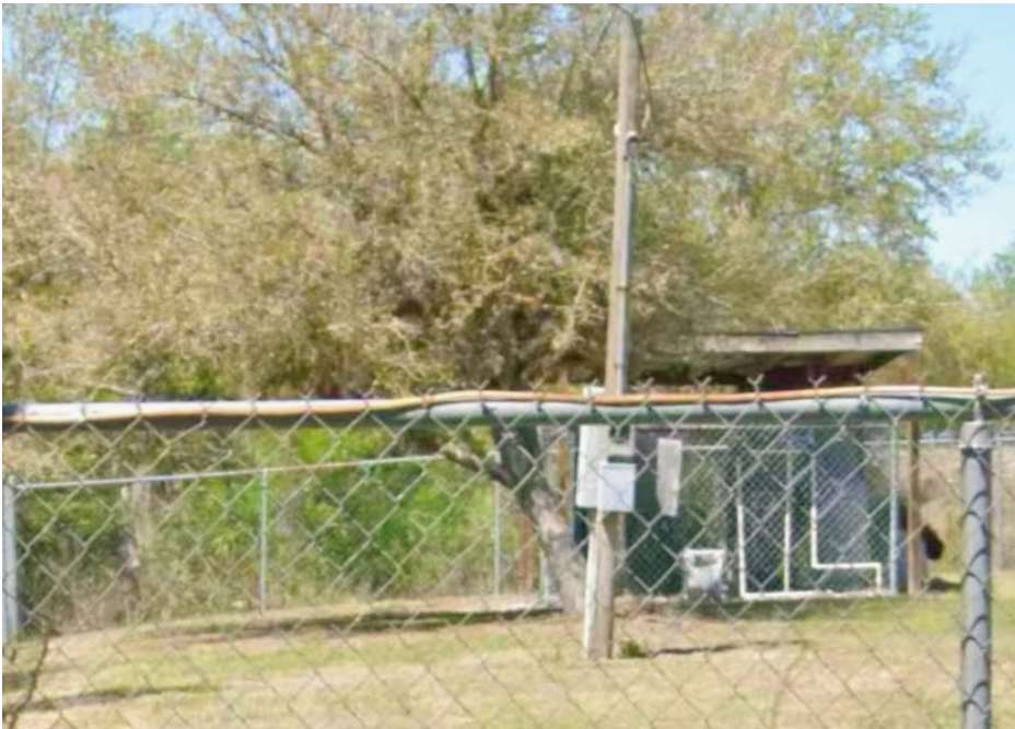
Figure 5: Brownville Park Well
