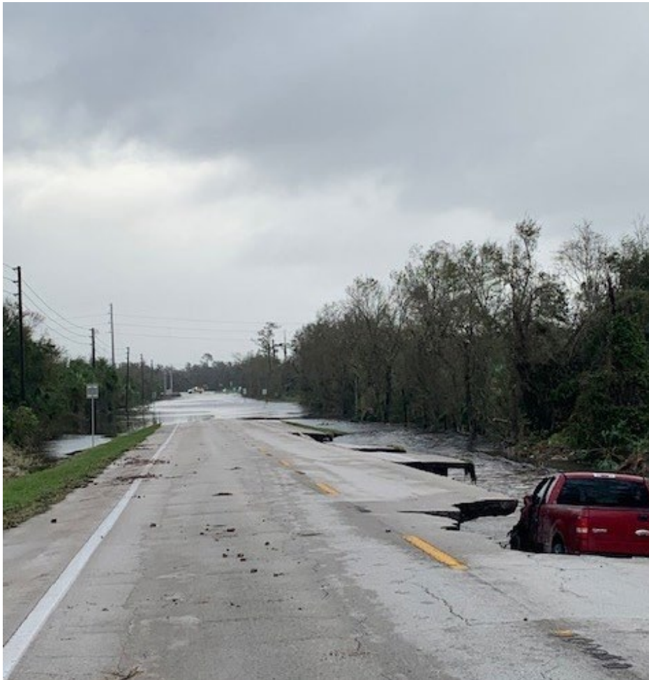
Figure 17: Severe flooding and road damage on SR 72 during Hurricane Ian
