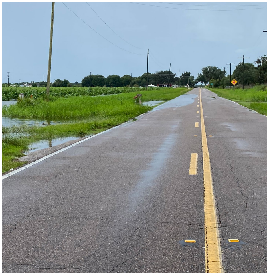
Figure 9: Flooding on West Main Street During Hurricane Elsa
