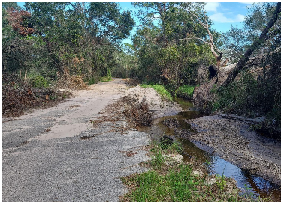
Figure 21: Storm damage and erosion along Highway 17, Zolfo Springs
