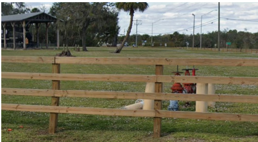
Figure 4: Public Water Systems Plant DDCV
