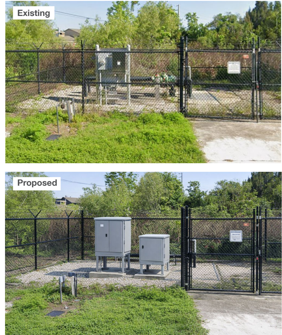
Figure 12: Visualization of Lift Station 30 Control Panels Protected with Dry Floodproof Enclosures
