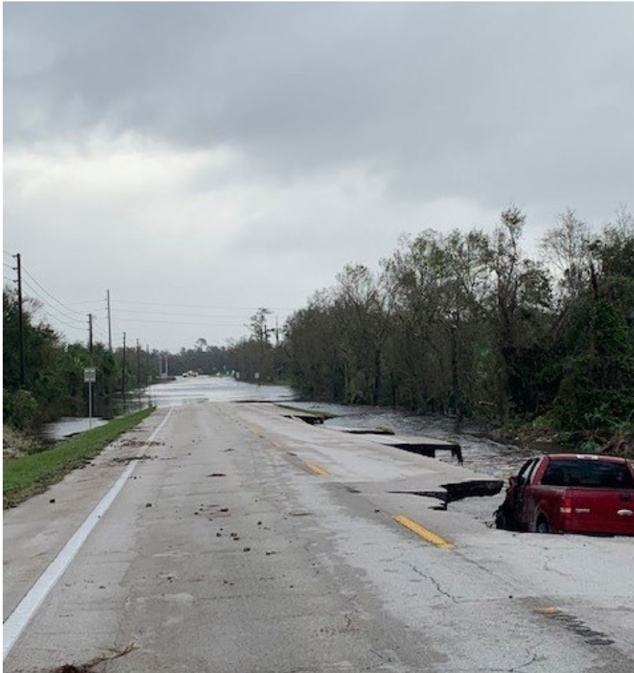
Figure 9: Severe flooding and road damage on SR 72 during Hurricane Ian
